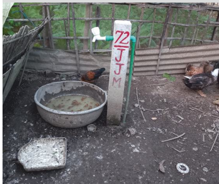
Photo 4 Swajaldhara ESR& Treatment Plant, retrofitted for Jal Jeevan Mission
