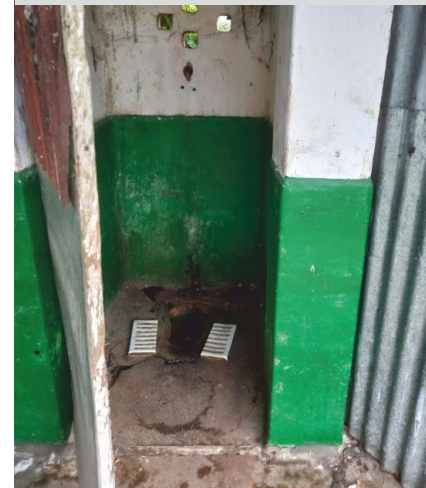
Photo 20 A Hospital Toilet without running water, in unhygienic condition
