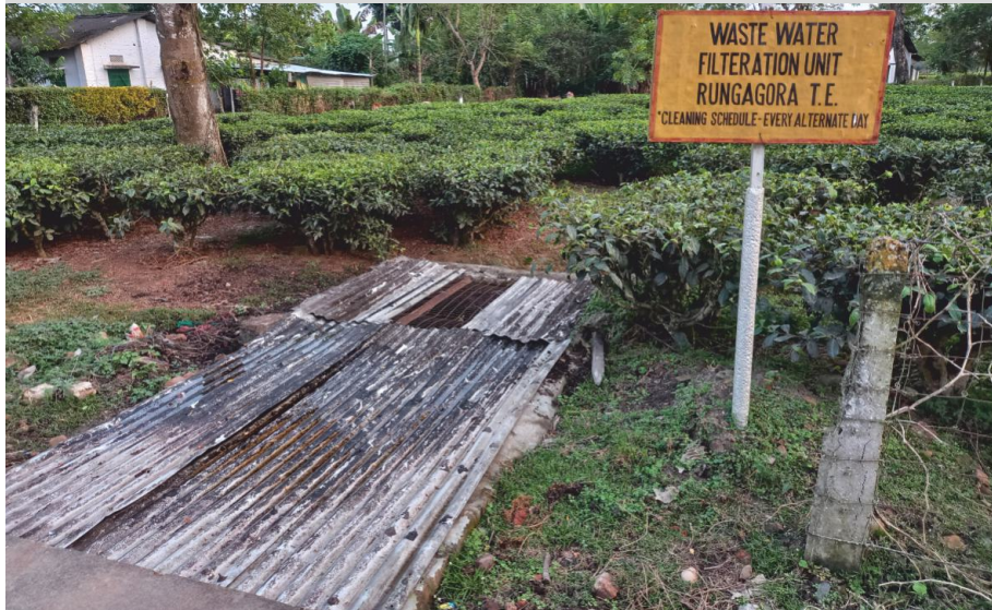
Photo 17 Wastewater treatment unit
