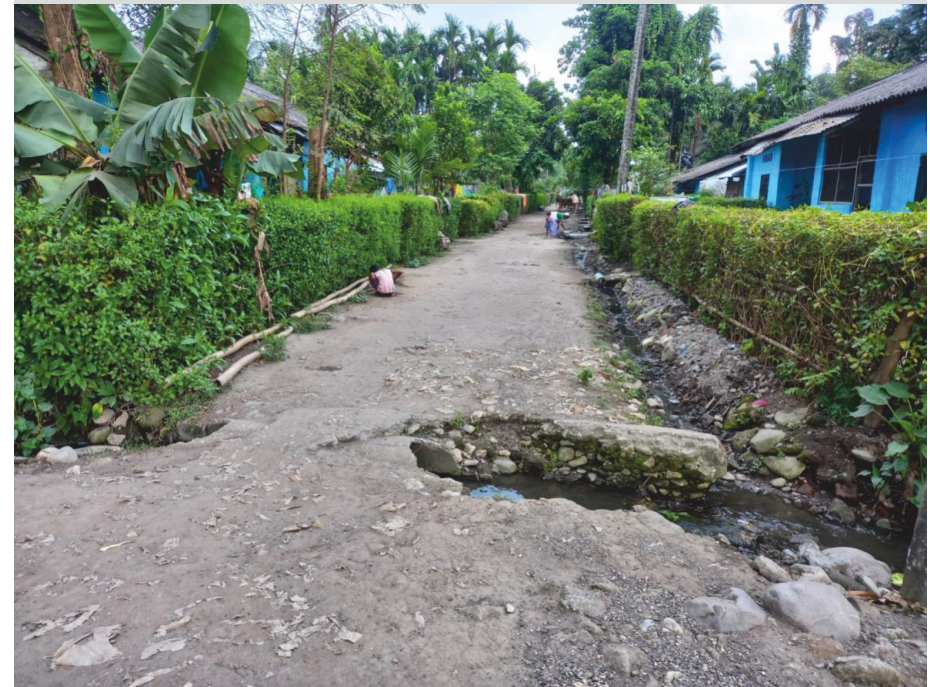
Photo 16 Free-flowing open sewage drains and broken culverts
