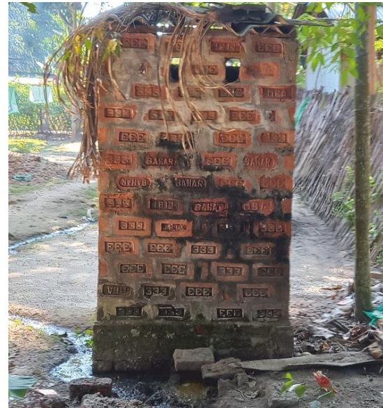
Photo 12. SBM Toilet with an open outfall
