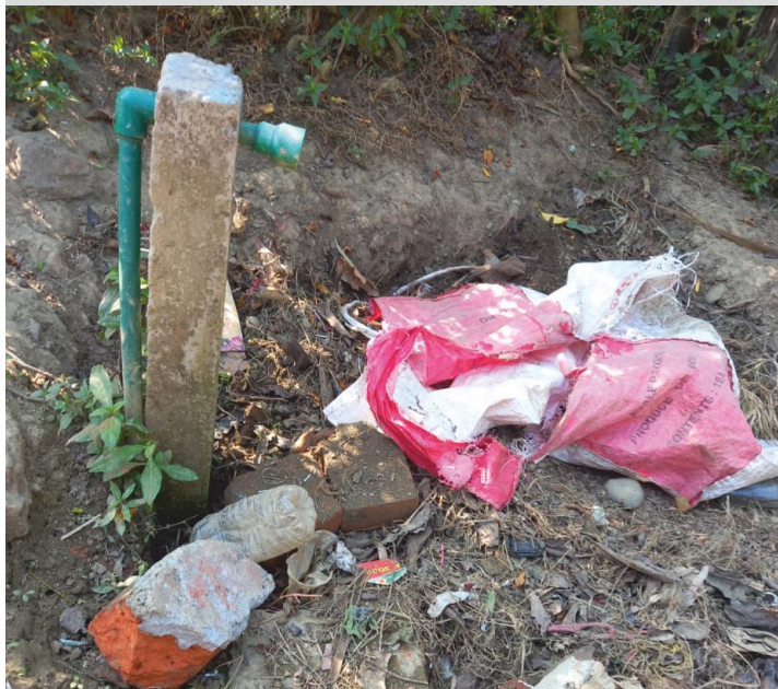
Photo 8 Broken taps, damaged standposts
