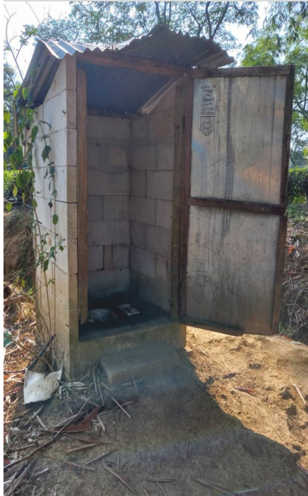
Photo 11 SBM Toilet without proper roof joints, door locks, water storage and leach pit cover
